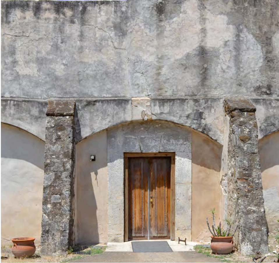
Plate 4. Main entry to the chapel. The C20 stucco cement was stained ca. 1963 and masonry buttresses were added ca. 1968 to several locations along the west and east elevations to provide 'historic' or 'antique' appearances. Photograph by author.
