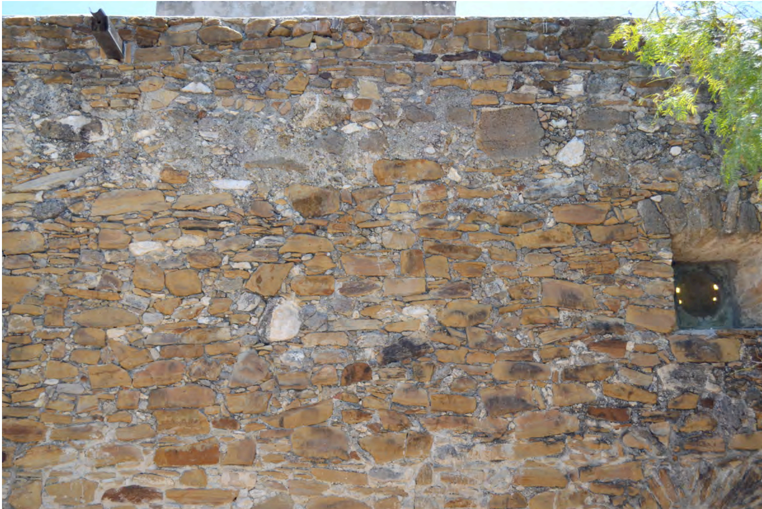
Plate B. North bay of west elevation showing top of wall with random stone repairs above ocular window. Photo by author.
