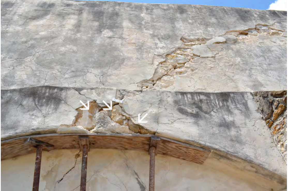
Plate 13. Detail above middle door in east elevation revealing arch masonry. Photograph by author.
