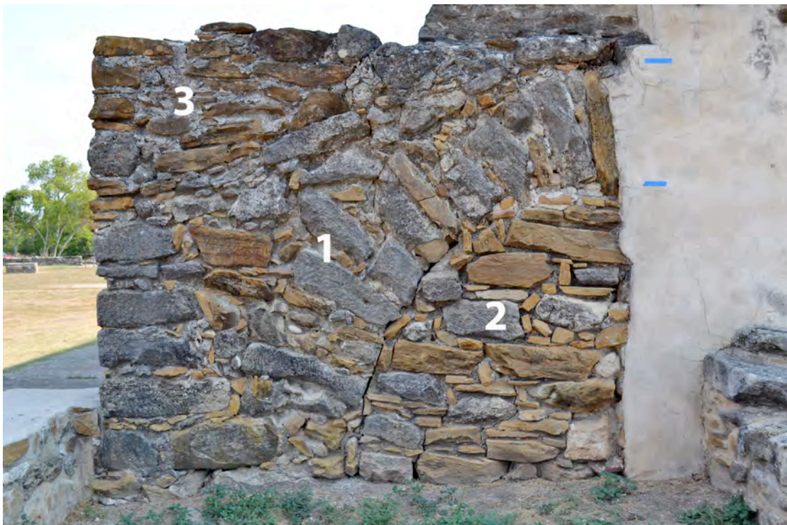
Plate 15. Buttress (1) at northeast corner of chapel that was blocked (2) and squared off for use as a wall (3). Photograph by author.
